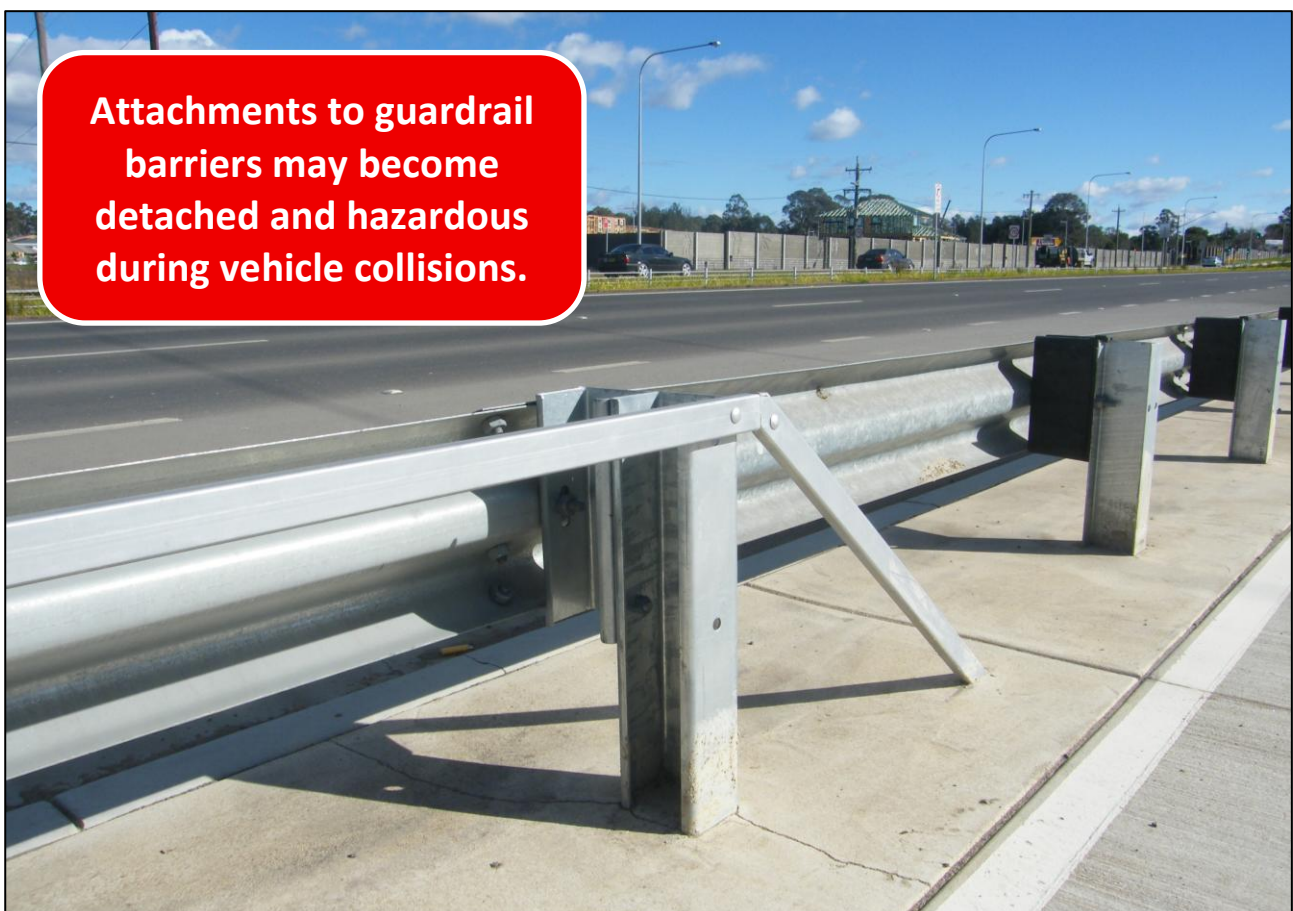
Figure 3: Pedestrian attachments to guardrail barriers can become hazardous during a vehicle collision.
