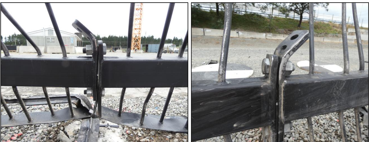
Figure 11: Unbroken M24 structural bolts.
