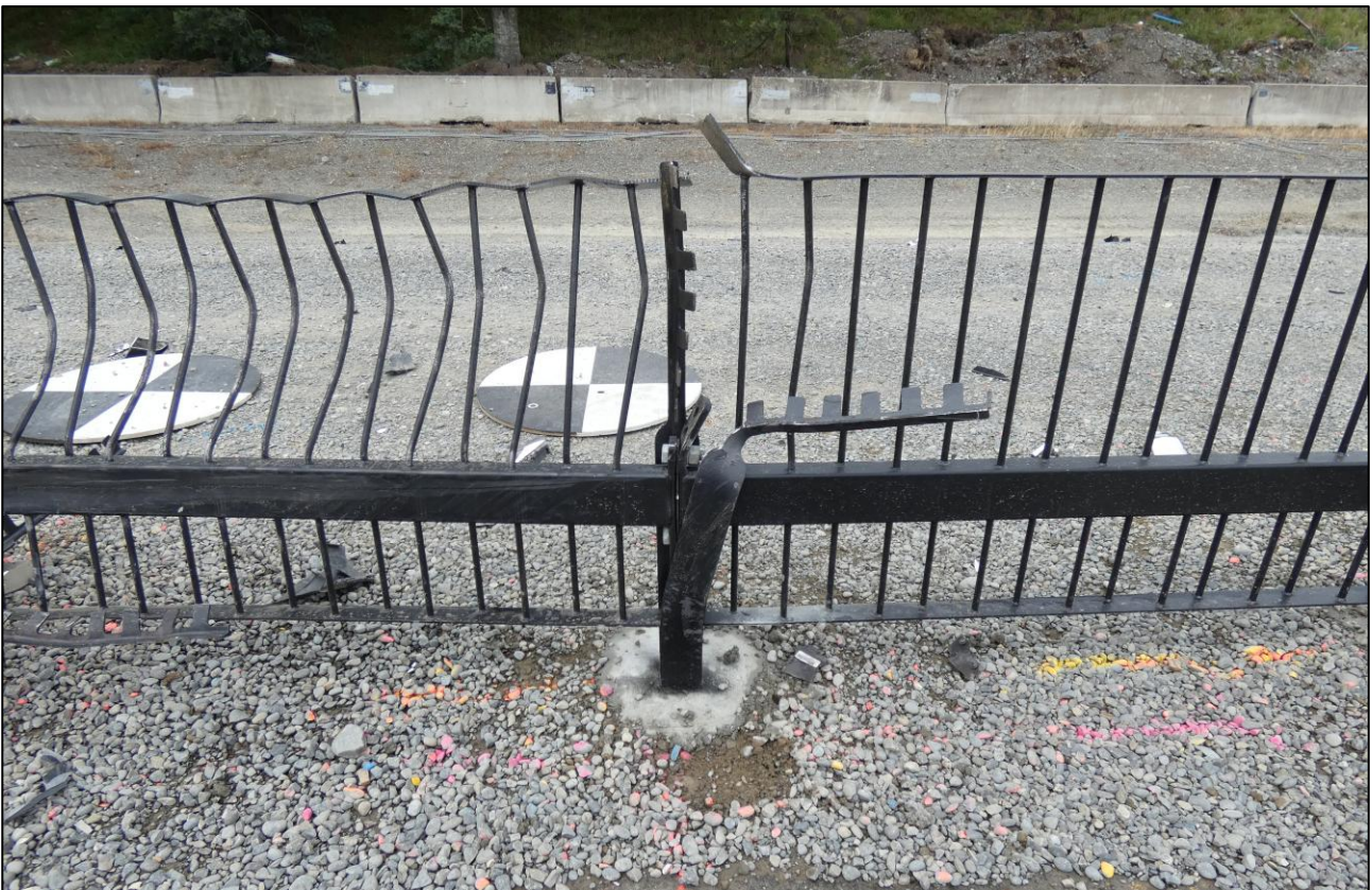
Figure 12: Damaged intermediate post.
